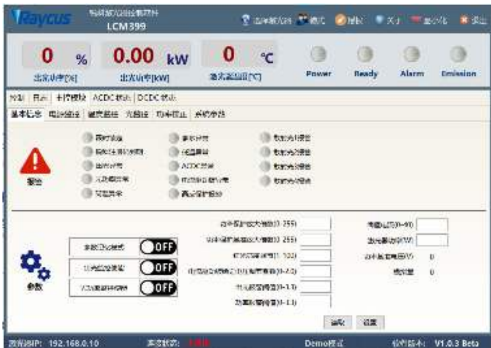
Figure 16 Main control module status information interface
